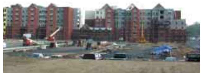
Hollowcore plank was specified for floor and ceiling elements in the new Lester Senior Housing facility in Whippany, N.J., due to its economics and fire resistance. The project is to be completed this fall.
